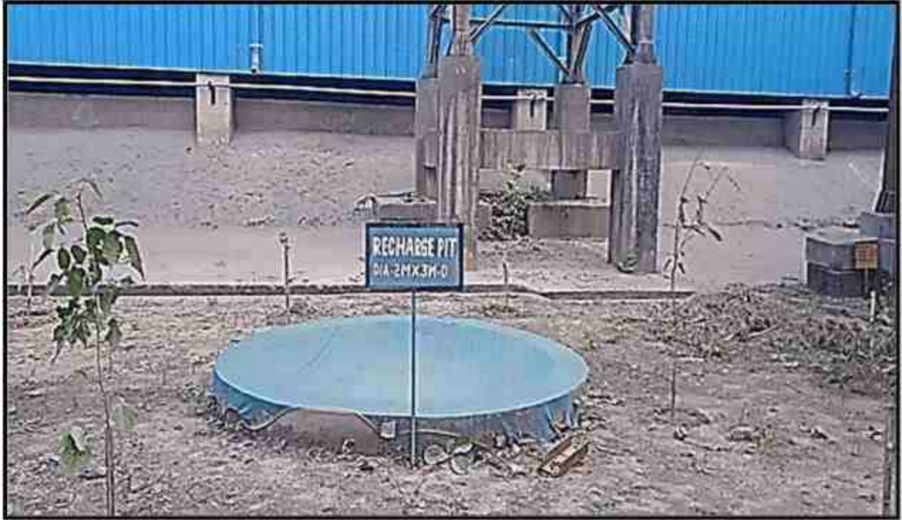
(2) Rain water harvesting recharge pit near Electrical load center
