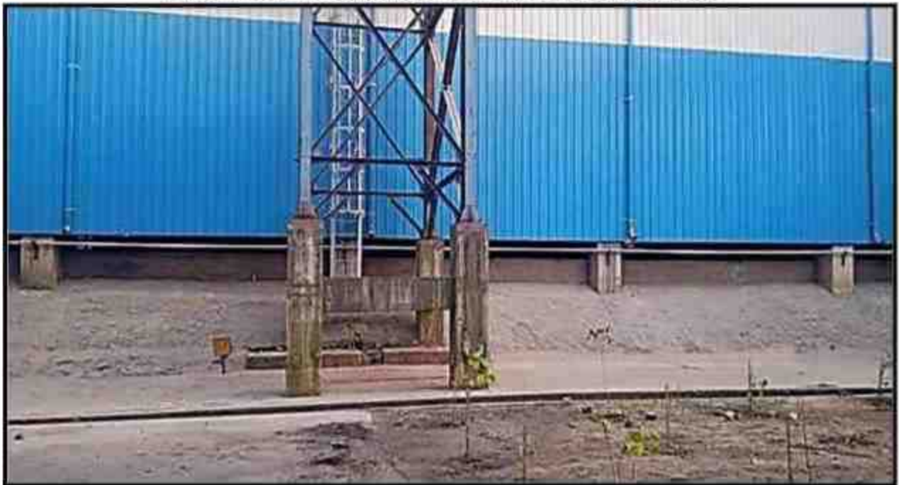
Rooftop Rain water collection pipe line, concreated drain connected to recharge pit near Electrical load center
