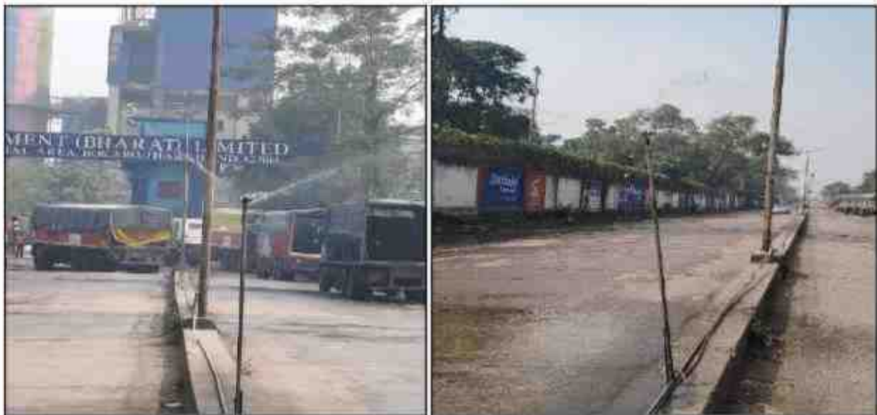
Fixed type water sprinkler installed plant main gate entrance road
