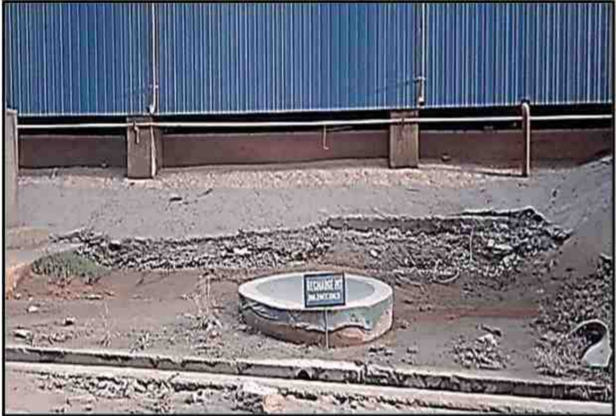
(3) Rain Water Recharge Pit with connecting drain near stacker reclaimers
