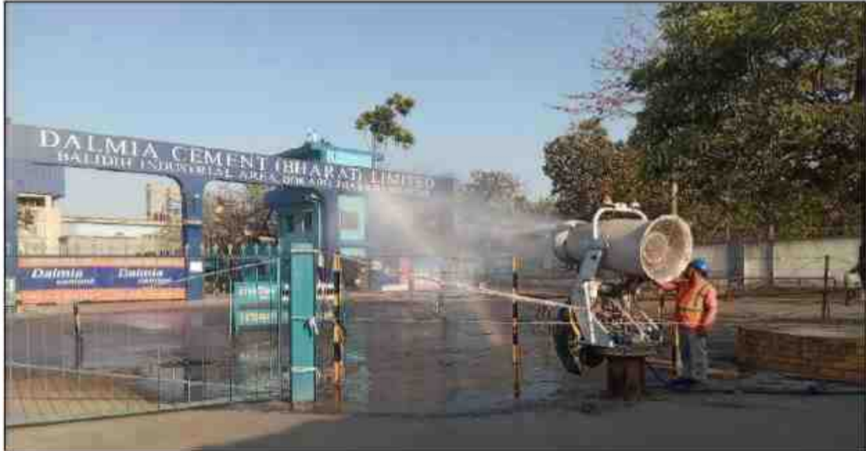
Water fog system installed in plant main gate
